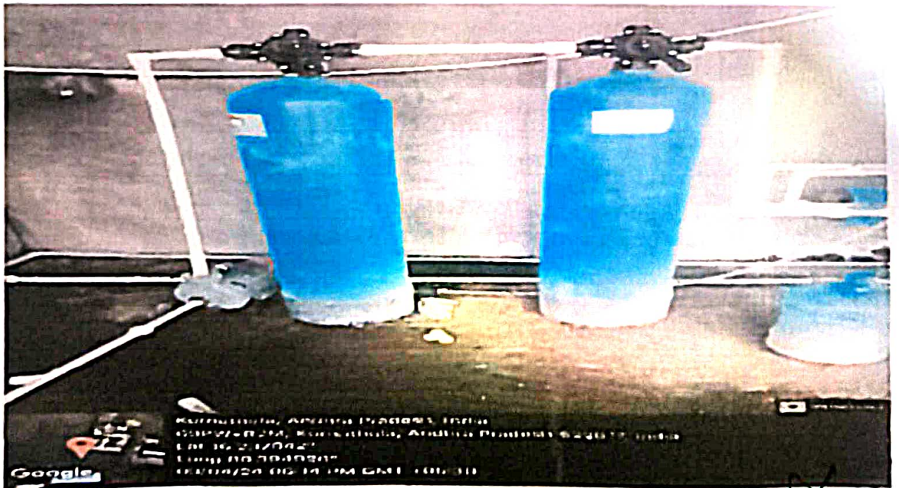
RO Water Plant
