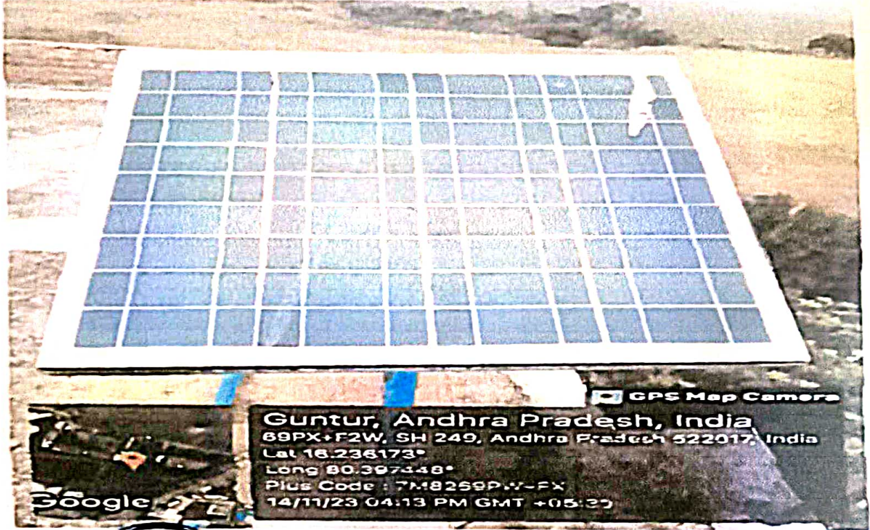
Solar Power in the Campus
